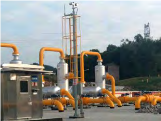
Natural gas border station
