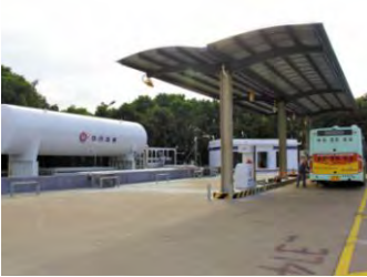
Natural gas storage station
